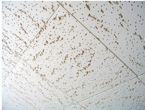
Asbestos containing ceiling tiles
