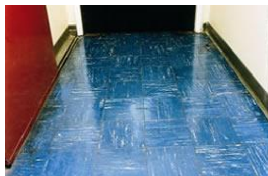
Asbestos containing floor tiles in a corridor
