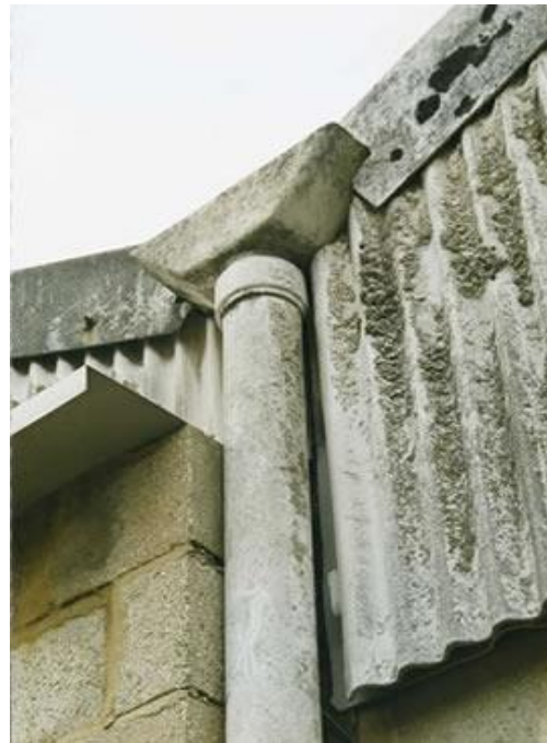
Asbestos cement downpipe, hopper and profile sheet
