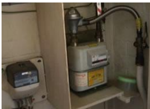
Asbestos panelling around a gas meter
